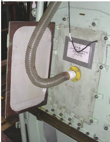
Sample of hose connection of dehumidifier system.
