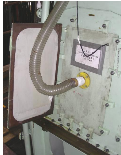
Dehumidifier outlet air taken from the crankcase
